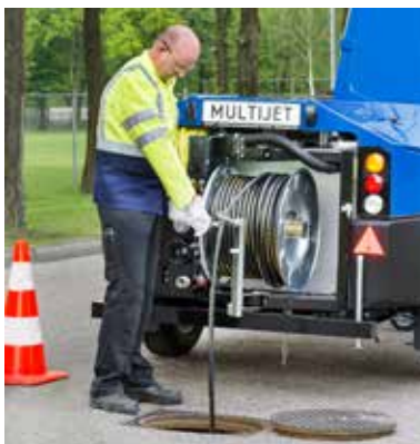
800 litres water on board
